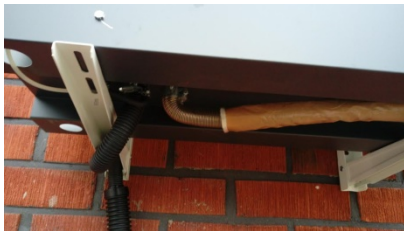
Picture 6. exhaust pipe and air-intake
